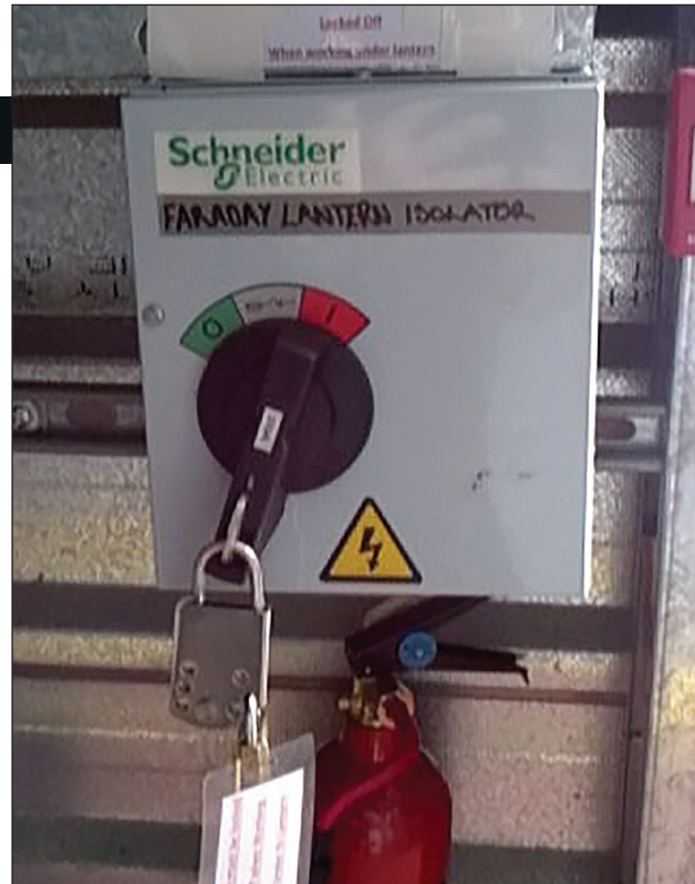
The Machine Room Isolator.
