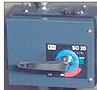
The Plant Room Isolator.
